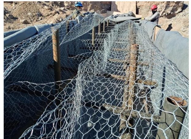
FIGURE 15 – Construction of temporary work with gabions and reinforcement tubing – Source: YPF SA
