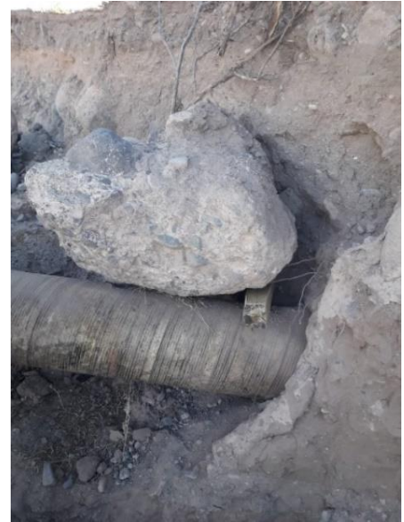
FIGURE 9 - Stone on the pipeline after the event - Source: YPF SA
