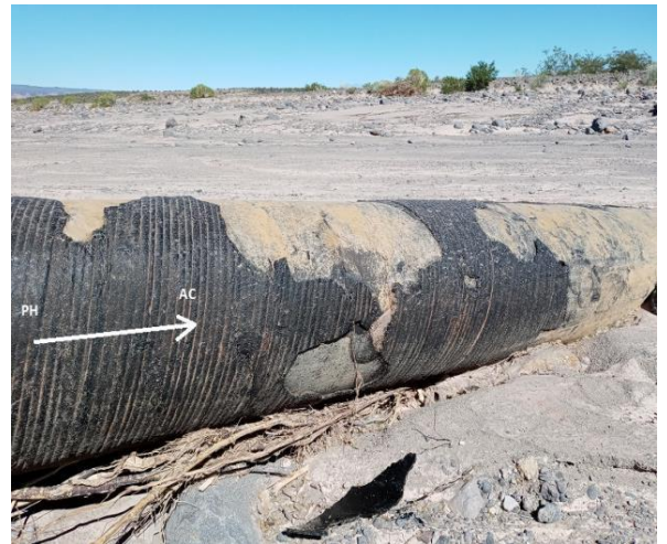
FIGURE 5 – Damage caused – Source: YPF SA
