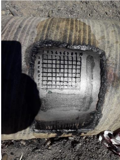
FIGURE 11 – pipeline damage assessment– Source: YPF SA
