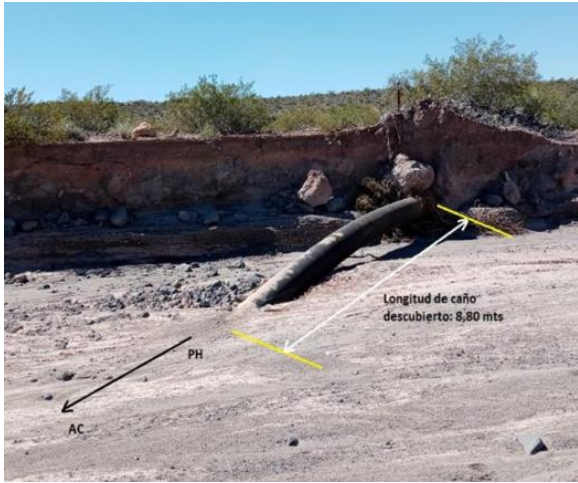
FIGURE 2 – Exposed pipeline– Source: YPF SA
