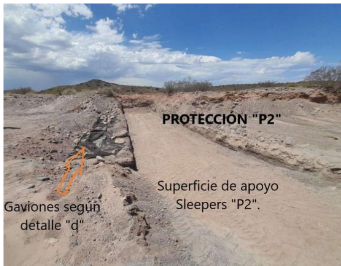
FIGURE 21 – Preparation of inclined surface for the placement of sleepers - Source: YPF SA
