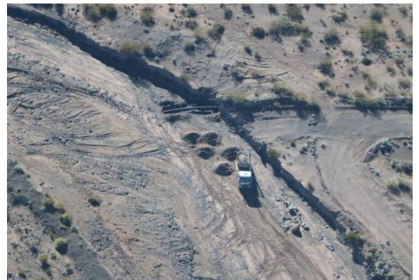
FIGURE 6 – Aerial view of exposed pipeline – Source: YPF SA
