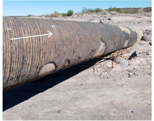
FIGURE 4 – Damage caused – Source: YPF SA
