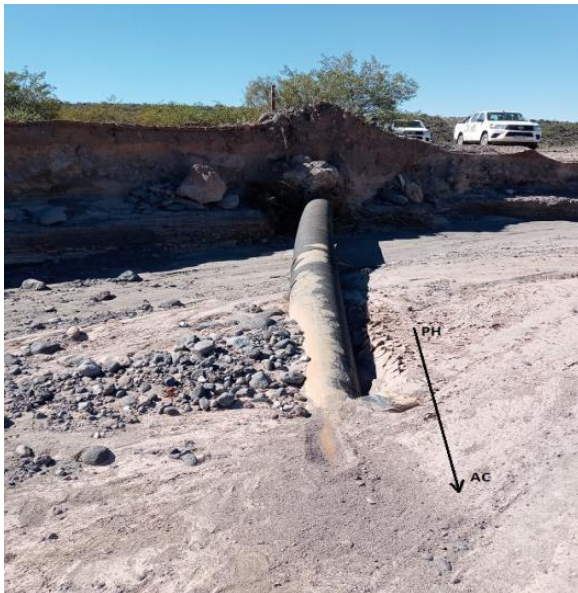
FIGURE 3 – Exposed pipeline– Source: YPF SA
