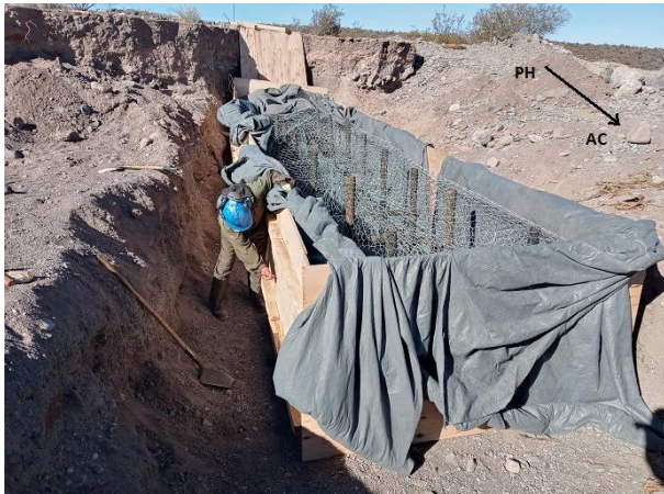
FIGURE 16 – Construction of temporary work with gabions and reinforcement tubing – Source: YPF SA
