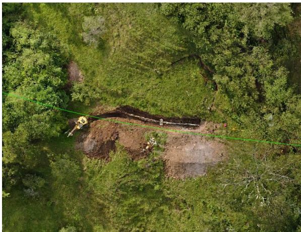
FIGURE 4. Cross-loading (hypothesis). Movement of the ground in a transverse direction to the alignment of the pipe, condition to bending. (Source: Own)
