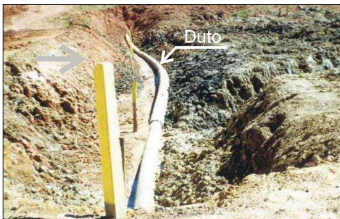
FIGURE 8: REAL CASE OF UNPROTECTED PIPELINE ON LOW CAPACITY FOUNDATION – LATERAL DISPLACEMENT.
