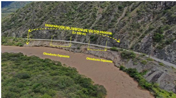
FIGURE 4: EROSIVO PROCESS THAT GENERATED THE DISPLACEMENT OF THE CHAMAYA RIVER BED TOWARDS ITS RIGTH SIDE, AFFECTING THE RIGTH OF WAY OF THE ONP.
