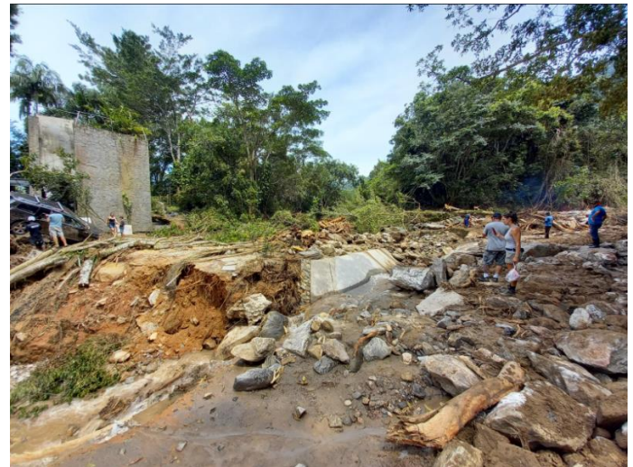
Figure 10 – picture of the concrete channel of hydraulic catchment 8 after the debris flow event of February 2023.
