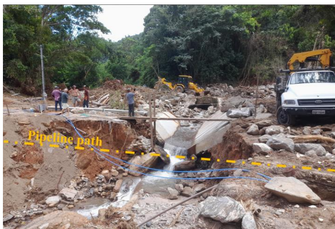
Figure 1 – Debris flow occurred due to the rainfall event of February 2023 in OSBAT, km 11+050, and the channel built an year earlier that protected it.
