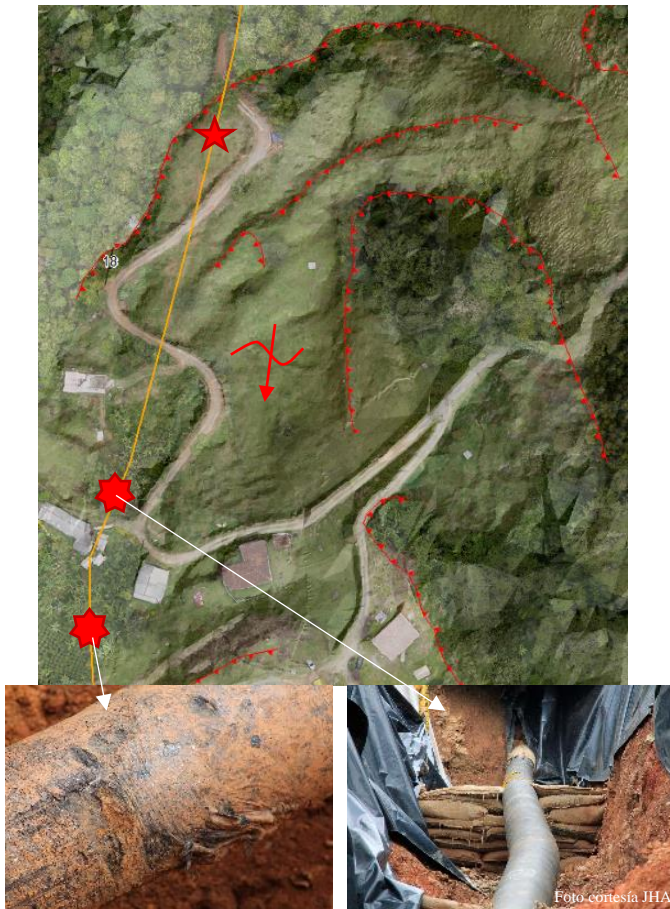
FIGURE 12: VULNERABILITY OF THE PIPELINE IN SECTOR 1
