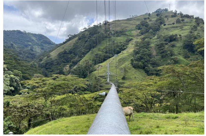
FIGURE 10: VULNERABILITY OF THE PIPELINE AT THE AERIAL CROSSING..
