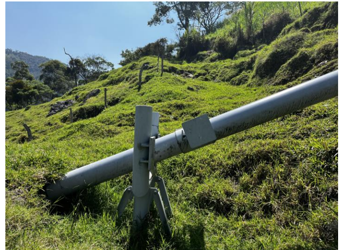
FIGURE 11: VULNERABILITY OF THE PIPELINE IN SECTOR 2 y 4
