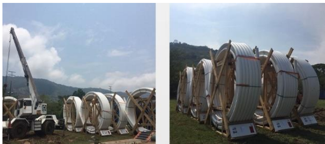
FIGURE 12. FLEXIBLE PIPE SPOOLS
