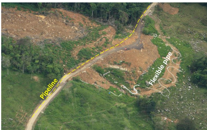
FIGURE 13. BYPASS IN FLEXIBLE PIPE (6").
