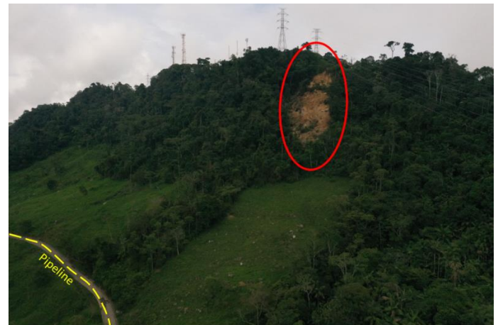
FIGURE 5. OCT. 2022. ROCK FALL LOCATED UPSLOPE OF THE ROW.
