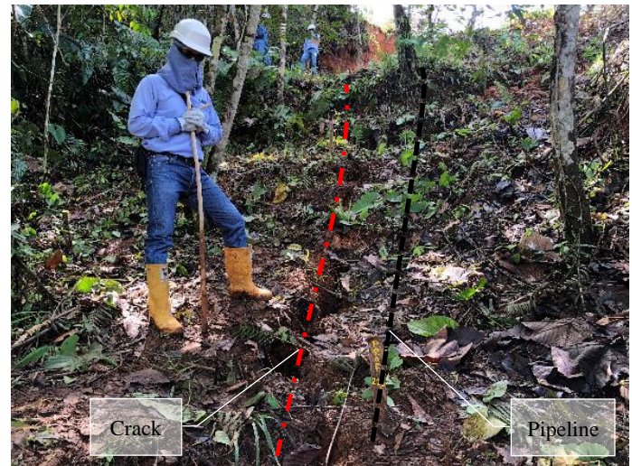
FIGURE 6. CRACKS IDENTIFICATION IN THE LANDSLIDE CROWN
