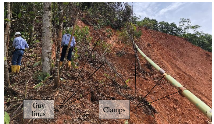
FIGURE 11. PIPELINE AND ATTACHMENT SYSTEM VIEWED FROM MAIN SCARP
