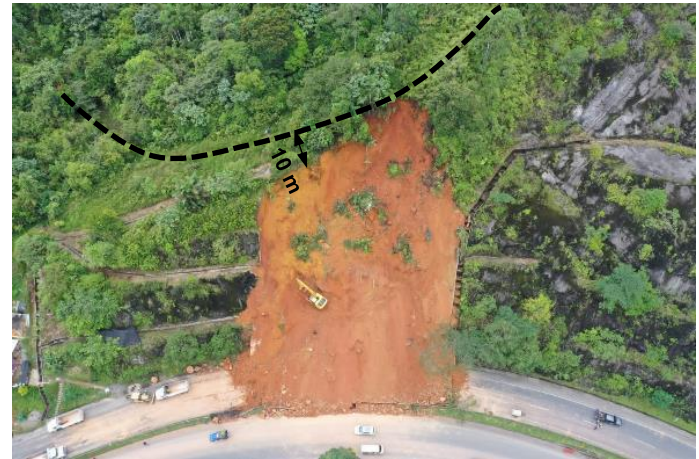
FIGURE 5. LANDSLIDE SCARP RETROGRESSION – SEP 2022
