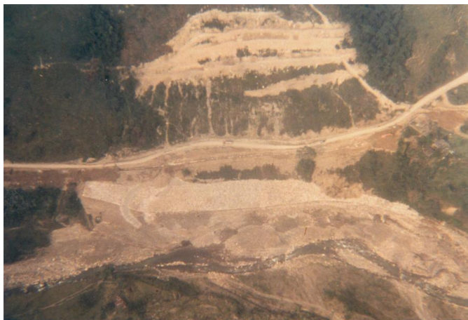
FIGURA 4: STABILIZATION WORKS CARRIED OUT BETWEEN 1994 AND 1997 TO PLACE PIPELINE IN INITIAL ROW (Photography by José Vicente Amórtegui IGL).
