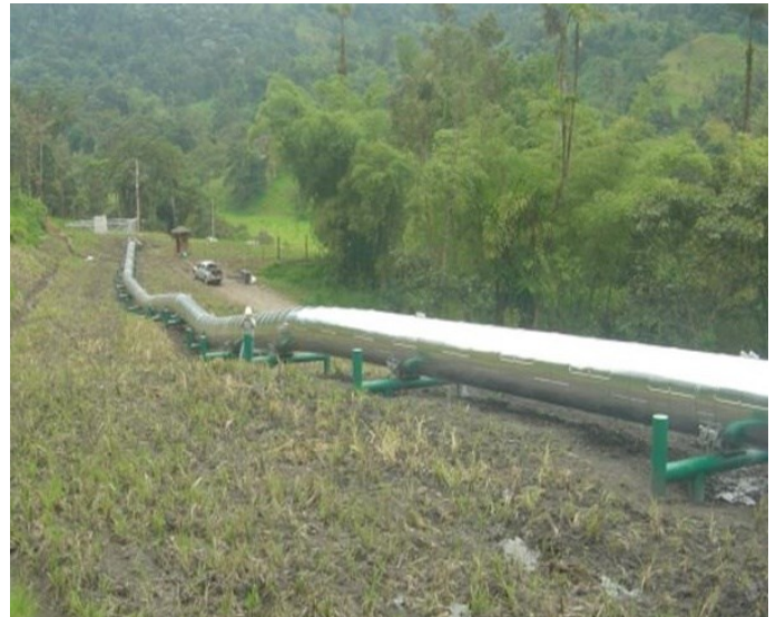
FIGURE 9: PIPELINE PLACED ABOVE GROUND ON VERTICAL SUPPORT MEMBERS TO ACCOMMODATE LATERAL SLOPE CREEP. (PHOTOGRAPH CREDIT: GUALBERTO CHIRIBOGA.)
